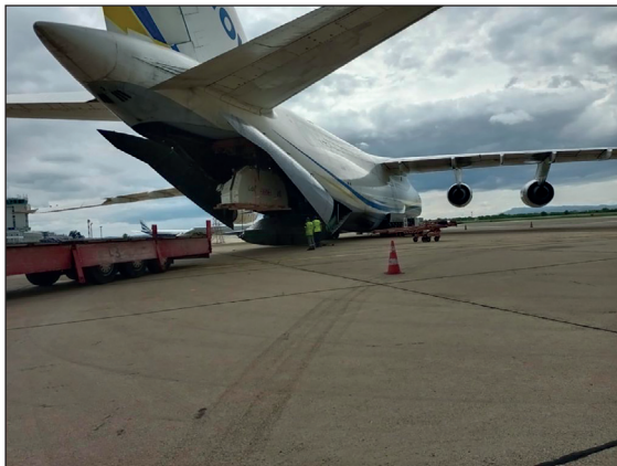
Views of the transportation of the plug in a cargo plane, its immersion at the site, and demolition of the concrete plugs. (Photos by EPM).
