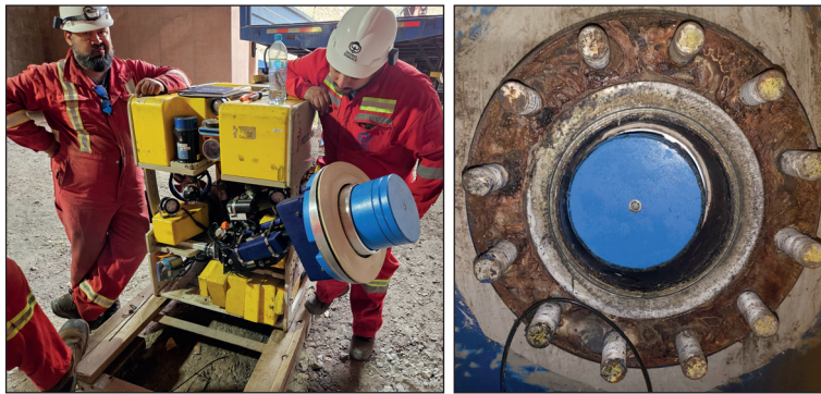
The ROV at Cheves, fitted with the plug (left) and downstream view of the installed plug (right).
