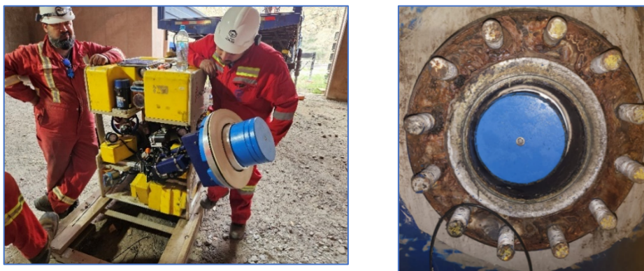
Figure 4-3: ROV fitted with the plug (left) and downstream view of installed plug (right)
