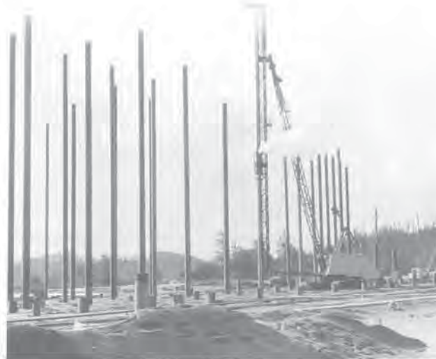
Driving pipe-pile caissons through compressible soils, 150-feet deep, at International Paper Co., Gardiner, Oregon, 1962.
