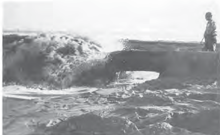
Crown Zellerbach, Richmond, B.C. – Placement on plant site of hydraulic fill dredged from the Fraser River, December 1954. Photo: Cyril Leonoff
