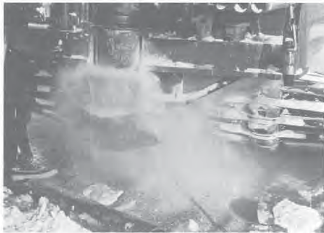
Mackenzie Valley Oil Pipe Line terrain evaluation – Drilling in massive ice lens with rotary drill, using air. Photo: Thomas Harper
