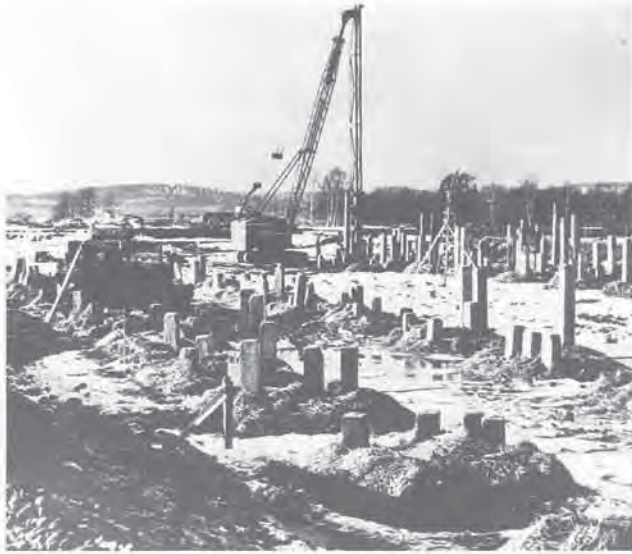
Driving precast concrete piles, Aktiebolaget Statens Skogsindustrier pulp and paper mill, Piteå, Sweden, 1961. Photo: Kjells FoTo AB
