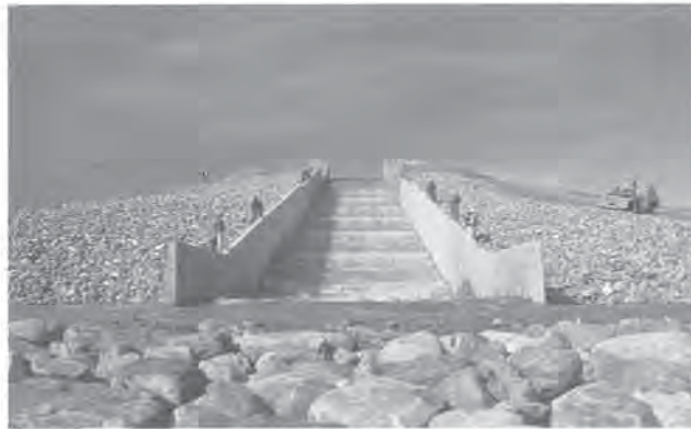
Inlet Chute showing the first flow into the reservoir from the St. Mary Canal.
