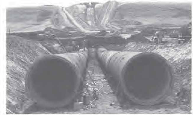
Inverted Syphon. Twin-barrel prestressed concrete pipes carry irrigation water 750 metres across the coulee, under construction August 1984.
