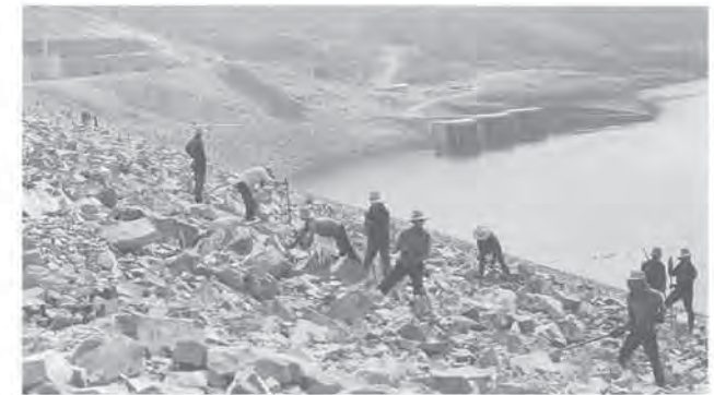
Sirikit Multipurpose Dam, Nan River, Thailand— Hand grading of riprap on upstream slope. Photo: Earle Klohn
