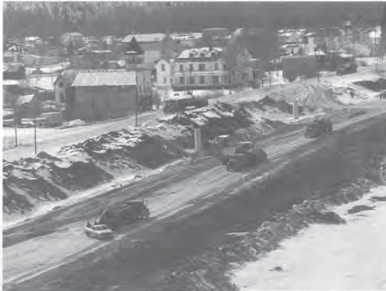
Construction of the Dawson City flood protection dyke, 1986–87 – Fill placement and compaction.
