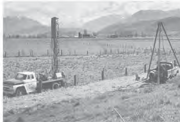
Drilling investigation and piezometer installation, Vedder Canal dykes, Fraser Valley, B.C., April 2, 1970.
