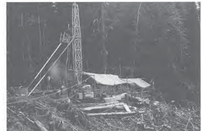
Ok Tedi project, Papua New Guinea – Lukwi tailings dam site investigation with helicopter-transported Longyear 38 diamond drill, ca. 1985. Photo: Mark Olsen
