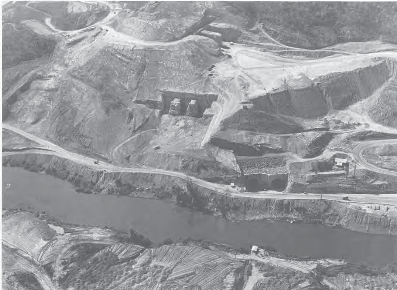
Sirikit Multipurpose Dam, Nan River, Thailand – Construction, ca. 1970. Photo: Royal Irrigation Department of Thailand
