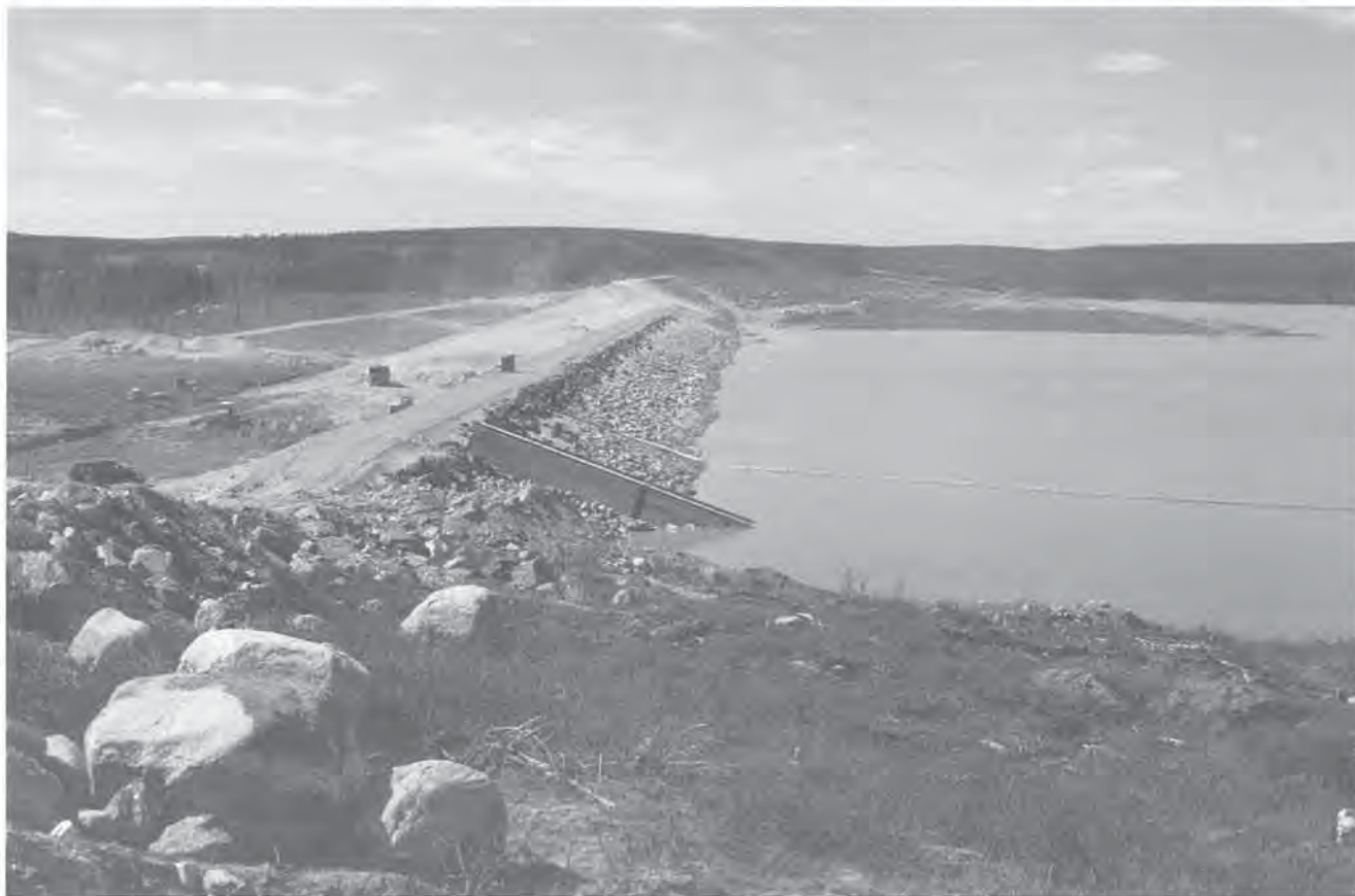
Quebec Cartier Mining Company Tailings Dam A, upstream view showing outlet box, Mount Wright, Quebec, June 1, 1989.
