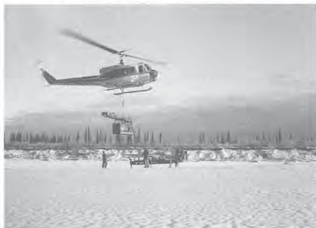
Bell 205 helicopter setting up heli-drill, Peel River crossing, Fort McPherson, Northwest Territories, 1970. Photo: Donald Davison
