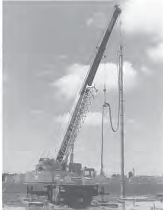
Densification test, 1981, of loose sand deposits by vibroflotation for Dome Petroleum, used in constructing artificial islands for oil exploration in the Beaufort Sea.
