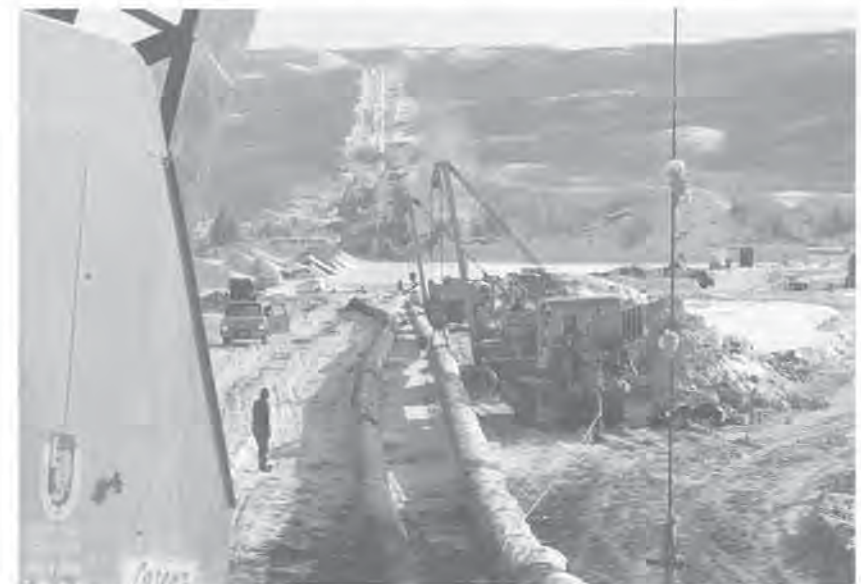
Peace River Oil Pipeline crossing Smoky River, Alberta. Photo: Matthews Photo Lab
