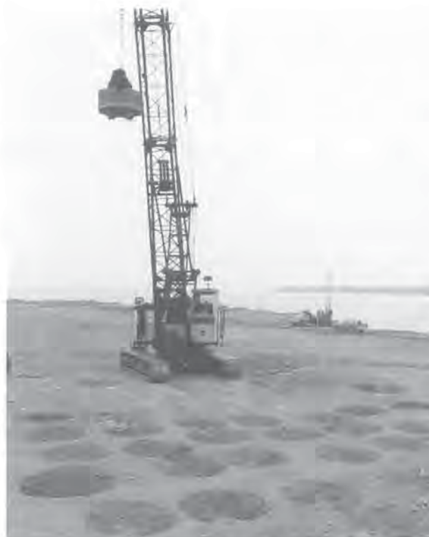
Dynamic compaction of rockfill with a 20-tonne weight, Duke Point, Vancouver Island, 1979.
