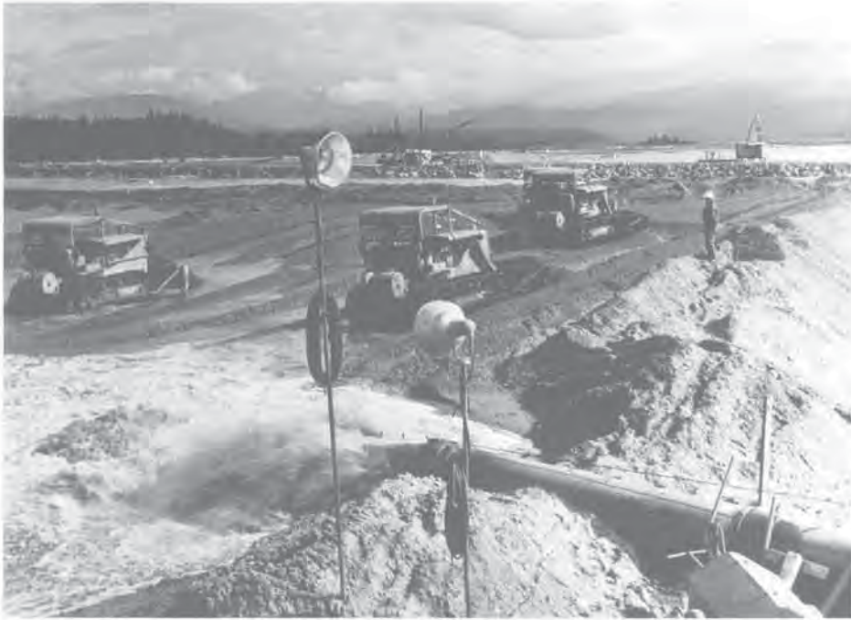
Aluminum Company of Canada, Kitimat, B.C. – Hydraulic fill placement at early stage of site development, spring 1952.
