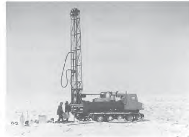
Drilling in permafrost with Nodwell carrier and Falling drill rig, Inuvik and Tuktoyaktuk, Northwest Territories, April 1972. Photo: Thomas Harper
