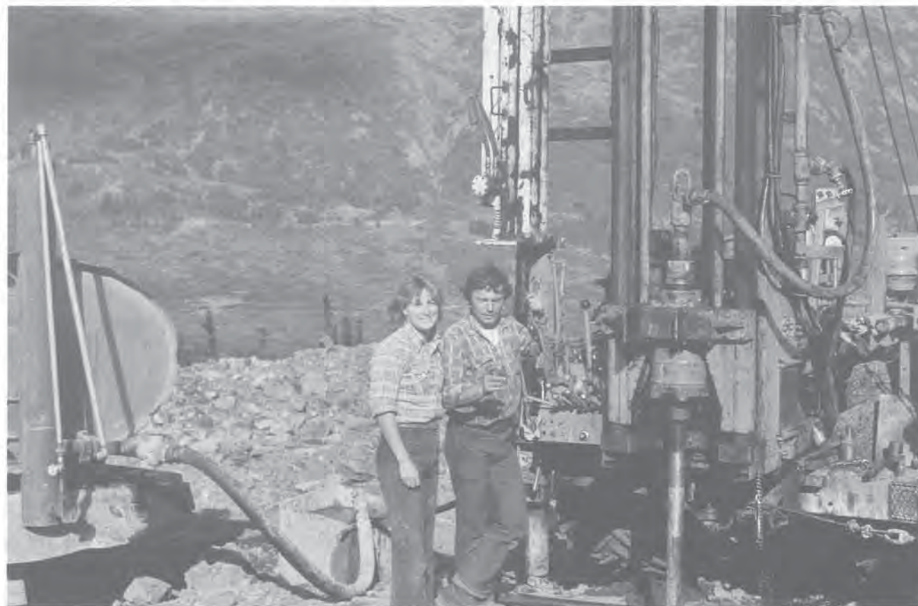
Adanac Ruby Creek Mine investigation, Atlin, B.C. – Engineer Peri Mehling and driller with rotary drill, August 12, 1980.
