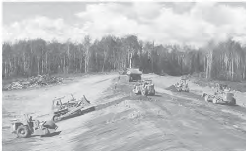
Reserve Mining tailings project, Minnesota, 1978-79 – Seepage recovery dam construction. Photo: Thomas Harper
