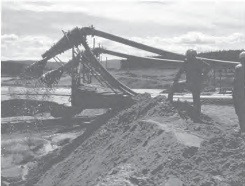
Hydrocyclones, Highland Valley, B.C. Photo: Earle Klohn
