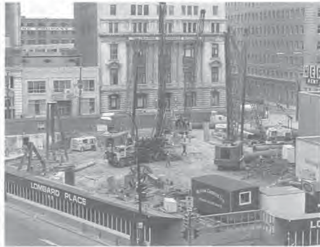
Caisson rigs at start of construction, summer 1967. Photo: Hugh Allan, Winnipeg Tribune
