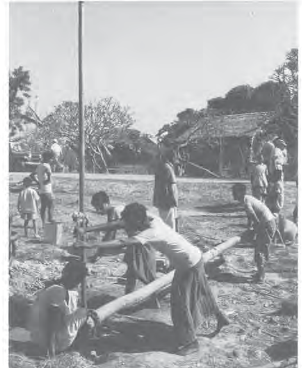
Water well drilling to 150-foot depth, village on Ganges delta, East Pakistan (Bangladesh), 1963. Photo: Charles Ripley
