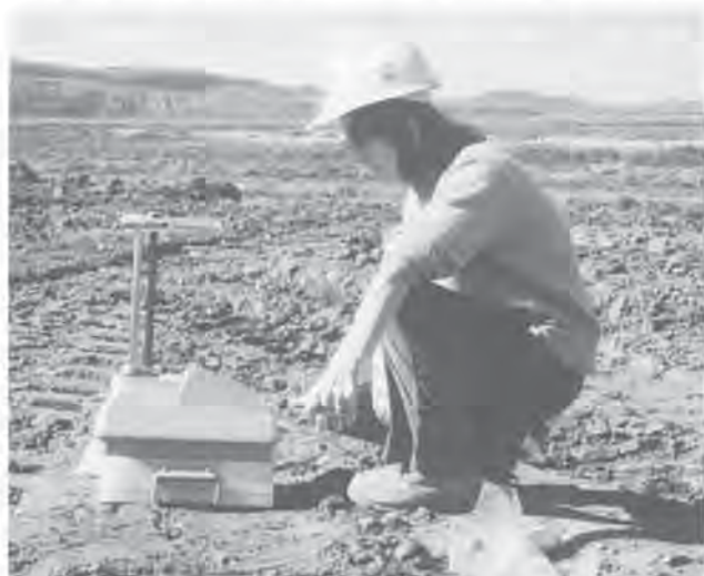
Reserve Mining tailings project, Minnesota, 1978-79 - Density testing of fill with nuclear apparatus.
