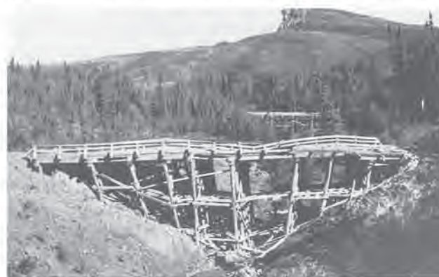
Structural damage of the Gardner Creek Bridge, Mile 358.4 Northwest Highway System (Alcan Highway), due to movements in the foundation soils, August 1951.
