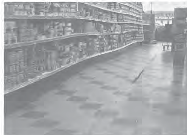
Uneven settlement of a supermarket floor built on peat, Fraser Street, Vancouver, B.C., 1952.
