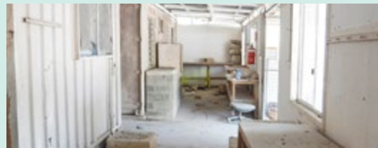
Run-down shelter prior to remediation
